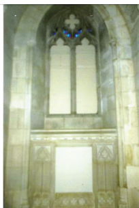
The Stonewall Jackson plasterboarded Windows and Inscription.
